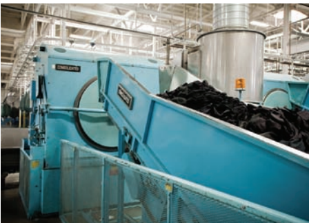
Shuttle conveyors automatically unload washers and load multiple dryers.
